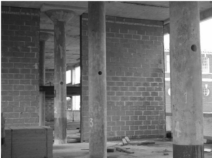
Figure 11. Ground floor office space during redevelopment, showing new block crosswalls, mezzanines and holes drilled to take steel supporting pins, 1999
