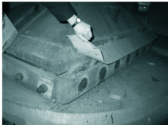
Figure 11. Top: Bearing of Blaues Wunder (Helas 1995, p.58), Middle: Arrangement of the bearings within the bridge system (Mehrtens 1900, Fig.141), Bottom: present Condition
