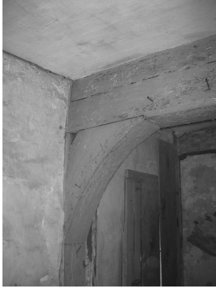
Figure 13. Exposed brace ( korbeel ) at Jan van Hoesen house, c.1750, Hudson, New York
