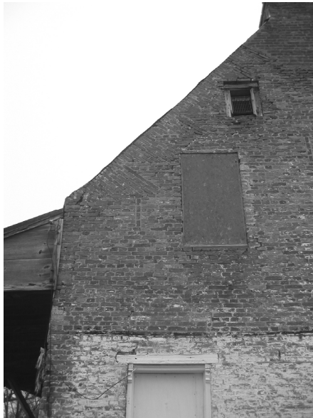
Figure 14. Brick Tumbling ( vlechtingen ) at the Jan van Hoesen house, c.1750, Hudson, New York
