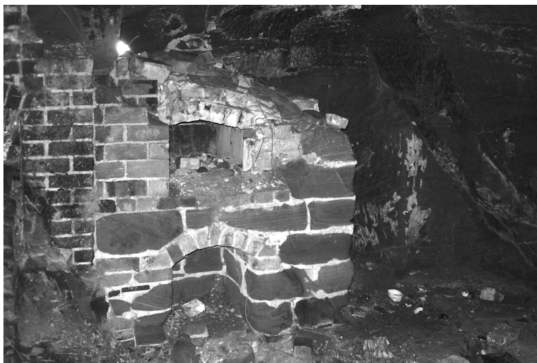
Figure 11. A Sandstone oven at Drakelow (west group) has only survived because of the isolated and overgrown location.
