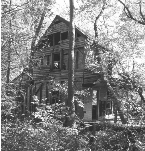
Figure 6. The deteriorated condition of the Hayes-Campbell Tenant House allowed easy access to the framing. CHAD Collection.
