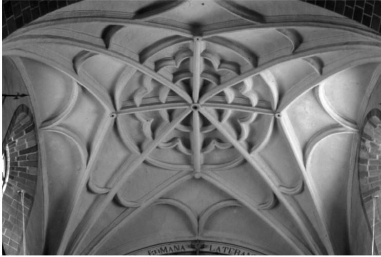
Figure 13. Francisco Domínguez de Chávez y Arellano, Cuzco, church of San Francisco, interior detail of rib vaulting, 1649 (photo: H. Rodríguez-Camilloni)
