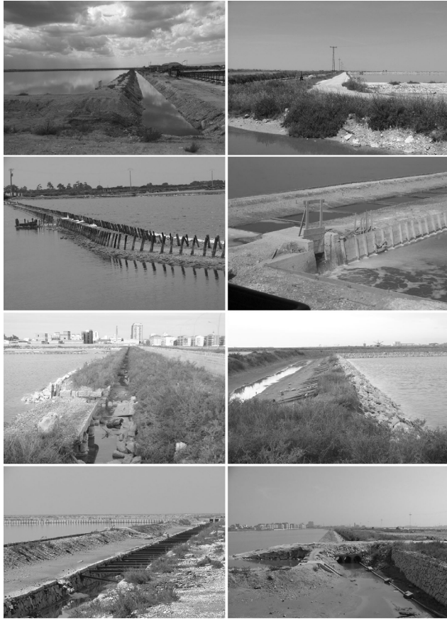
Figure 2. Different types of embankments. From the 'soil movement' to the built structure
