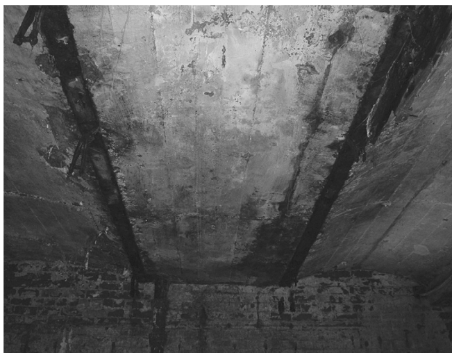
Figure 6. Concrete jack-arch floor supporting the yard of the Myrtle Road houses (March 2004).
