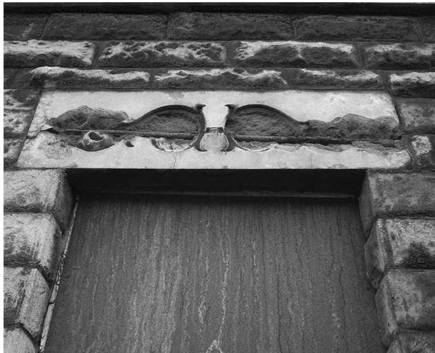
Figure 2. Lintel of Queens Road house, showing corrosion of internal reinforcement (March 2004).
