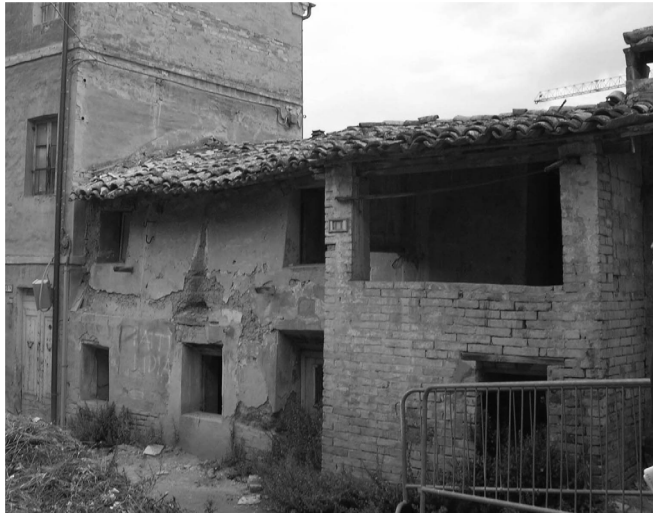
Figure 7. A masonry foundation is visible low on the left. Note also the external masonry stair to the right, the overhanging eave and the surface erosion on that part of the wall unprotected by the roof.
