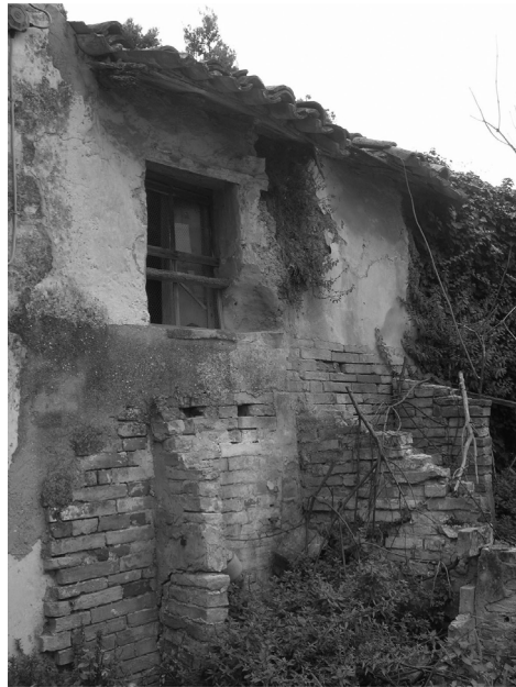
Figure 2. An earth building abandoned by its owners
