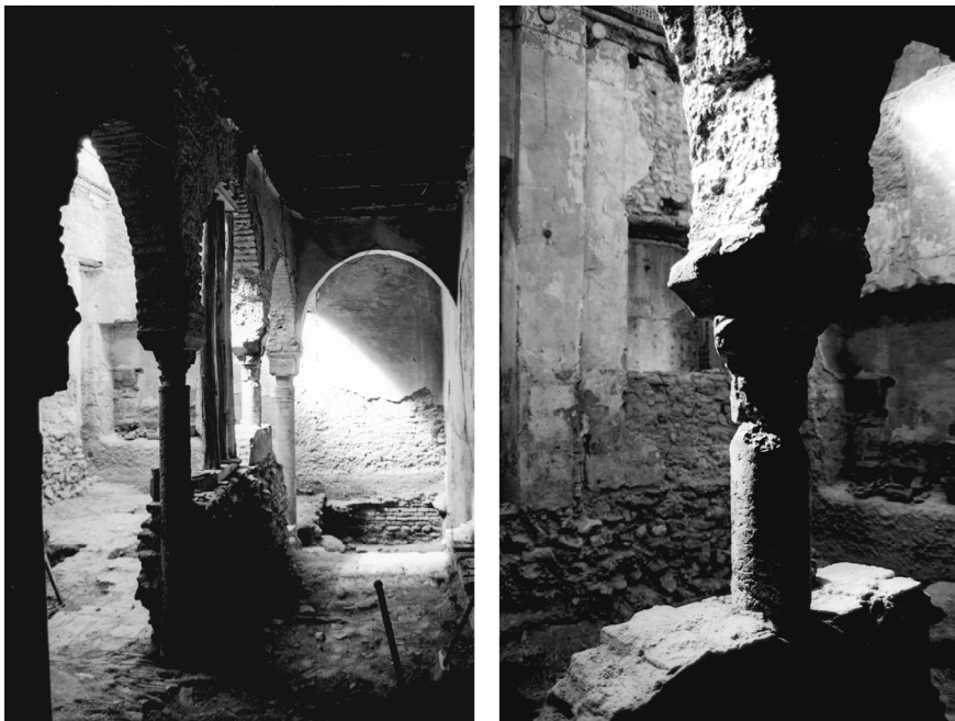
Figure 4. Images of the demolition to clear the Arab baths from domestic additions
