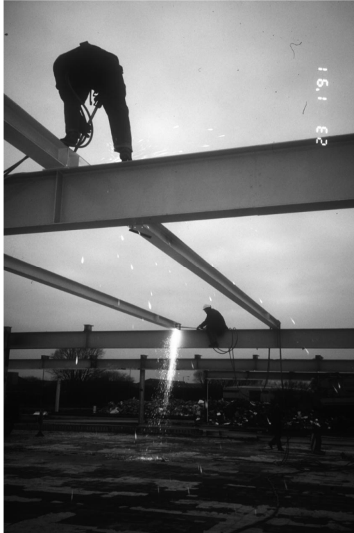
Figure 5. Site welding, that was rare at the time, was exploited by Hunt from the very beginning of High Tech.
