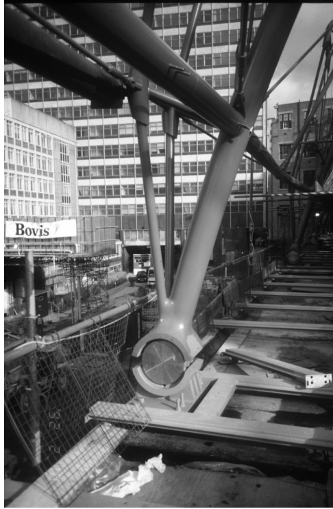
Figure 12. The weldable cast steel nodes contributed greatly to the elegance of the final design for the Waterloo Terminal.
