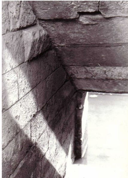
Figure 5. Unfinished outer face seen down the second straight flight of stairs of the Square well
