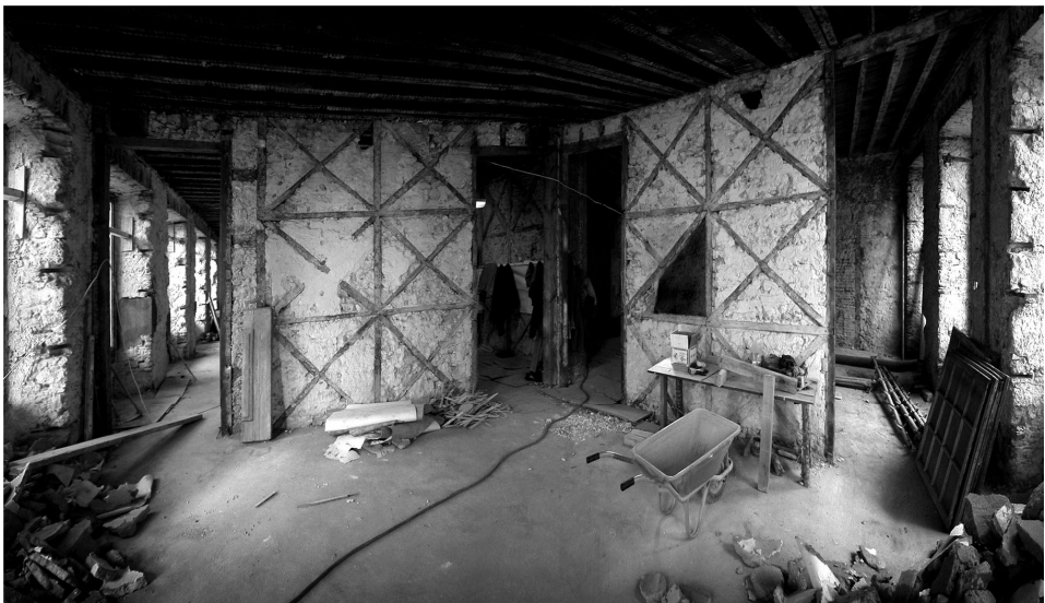
Figure 13. Interior of late 18 th Century building with Pombalino walls revealed during renovation work in 2003. This example has does not have the gaiola frame extending into the exterior masonry.
