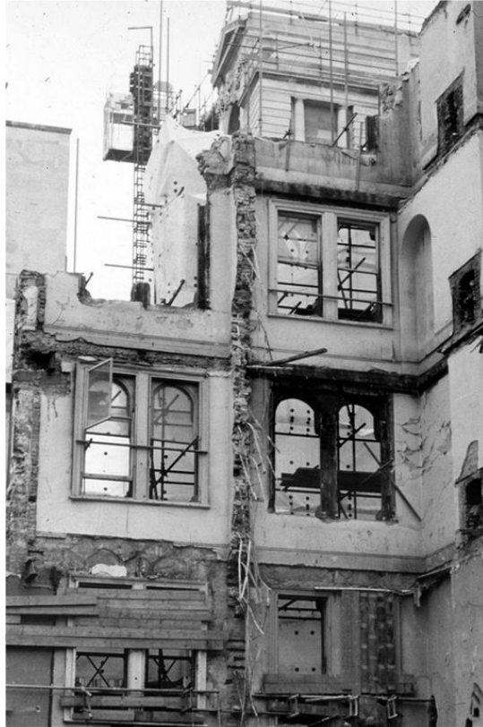
Figure 12. Back of front wall of buildings c1870 in Poultry, London in course of demolition showing quantity of hoop iron bond connecting front & party walls
