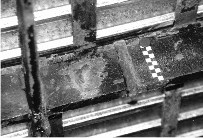
Figure 12. South-east pavilion: damage dated from the World War II
