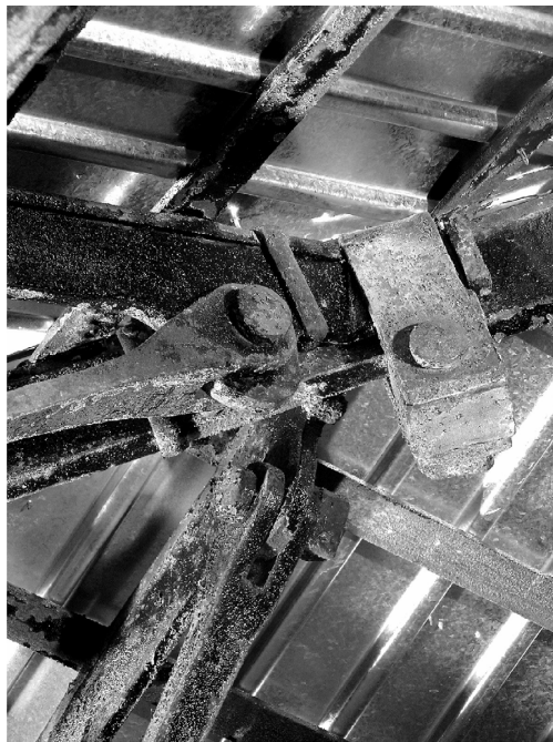
Figure 7. Clamp connection between jack and hip rafter in the pavilion roof frames
