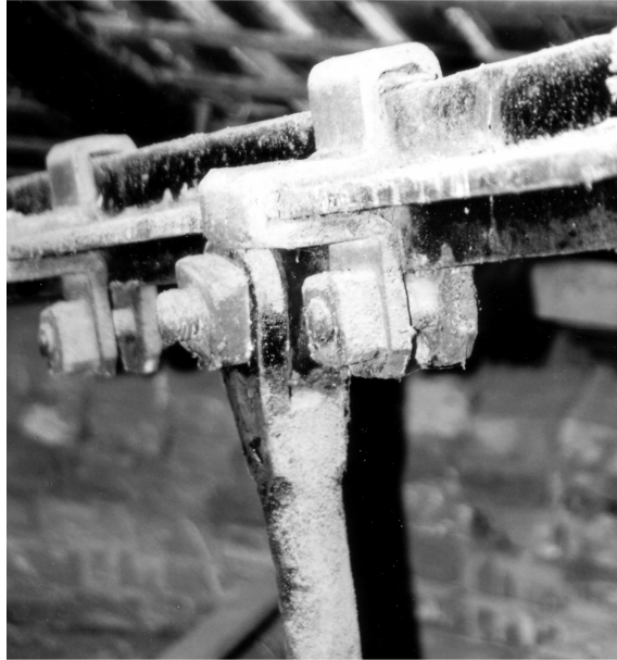
Figure 8. Stabilized upper chord of the support truss in the pavilion roof frames
