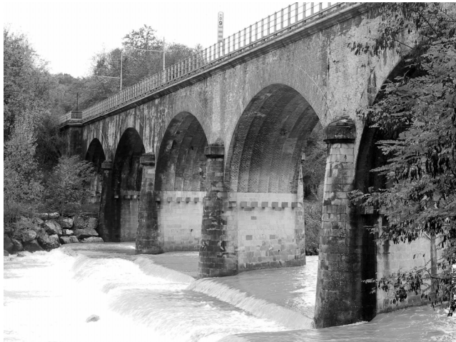
Figure 13. The bridge in Lama di Reno after sixty years since the rebuilding
