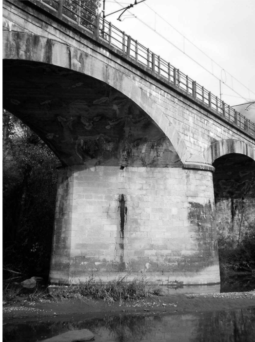
Figure 15. Bridge near Vergato on Porrettana railway. Detail of oblique vault rebuilt with concrete.
