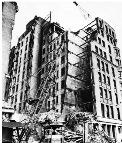
Figure 2. The Gladstone Hotel (1890) in Philadelphia: bearing walls and steel beams visible after demolition of floor arches and an outside wall. (HABS/HAER http://memory.loc.gov/ammem/collections/habs_haer/ )
