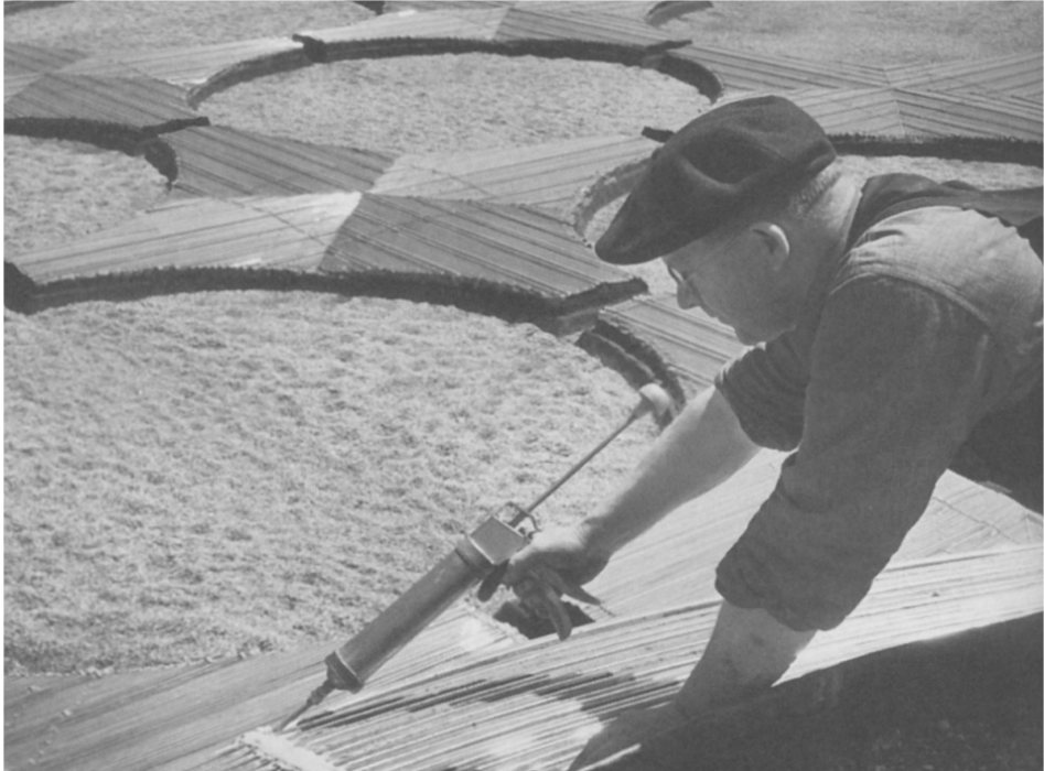
Figure 10. Workman caulking Pyrex tubing, skylight on roof Great Workroom. (Lipman 2003, p. 80, fig. 81)
