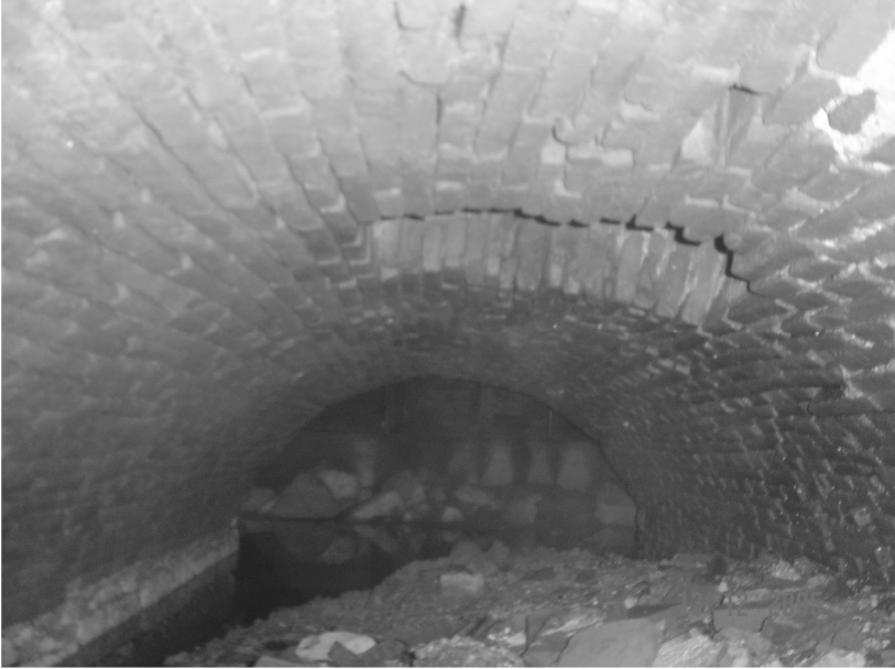
Figure 12. Current state of what may be Carnicerías Bridge (Author's photograph)
