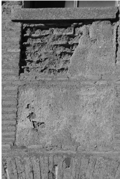
Figure 10. Construction detail of the same building showing the adobe filling the gaps between the bricks.
