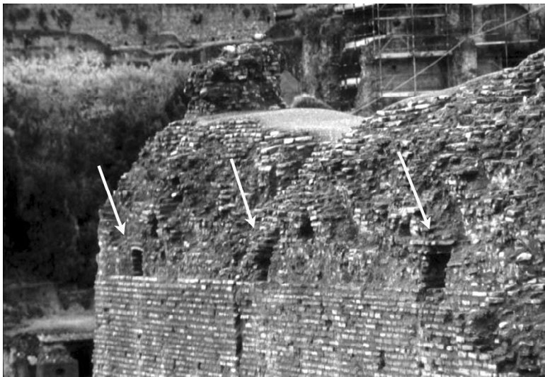
Figure 9. Southwest perimeter wall, interior. The rectangular holes are clearly visible and are built along the spring line of the vault. They are marked by a course of bipedales , connected with the reference tubes. Each cavity is 45 centimetres wide, 35 centimetres high and 124 centimetres deep and have bipedales on top.
