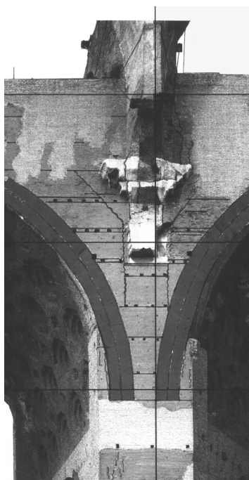
Figure 4. Photogrammetric image. Central nave: face of the upper part of the supporting wall of a pair of barrel vaults, to which was attached one of the columns supporting the cross vaults over the central nave. The compression loads on the part of the brick-faced walls supporting the cross vaults (under the entablature) were proportionally much greater than those of the lateral segments. This clearly differentiated treatment, designed to avoid uncontrolled structural cracking, reveals a remarkable amount of experience gained in the design and construction of vaulting systems.
