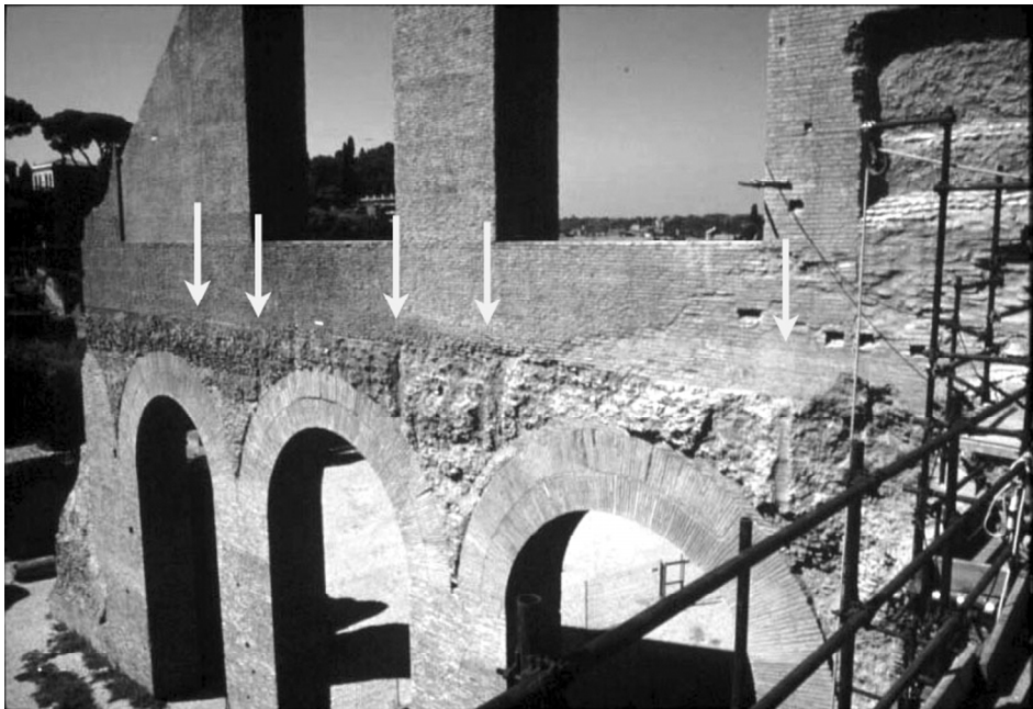
Figure 6. East end. Remains of terracotta tubes used as reference devices on the face of the walls and along the edge of the cross vaults.
