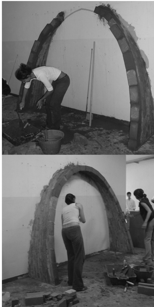
Figure 2. Assembling stages of the Nubian Vault: the first inclined layers are not complete, only after a certain number of layers the catenarian arch may be closed.
