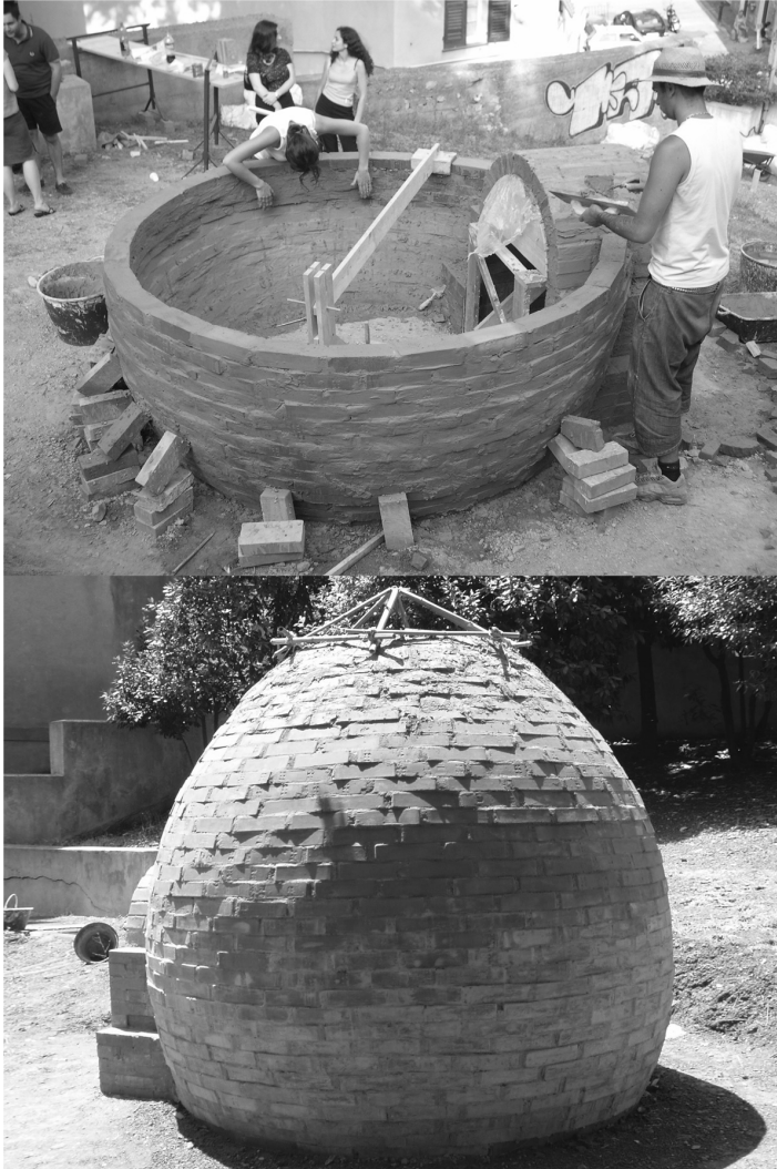
Figure 3. Assembling stages of the Ogival Dome: thanks to the special compasses being used, the largest diameter of the dome is above the ground level and the section is cuspidated.
