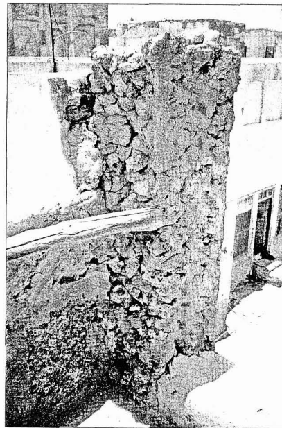
Fig. 15 Construction of Roof Badgir. The inner/upper farsh panel has collapsed, but the supporting pole is still in place.
