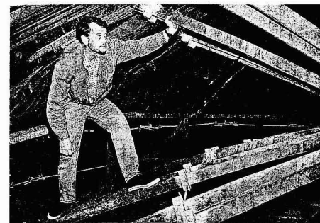
Fig. 5 Kazan Cathedral: the braces between the outer and inner ribs of the dome (showing also reinforcement introduced in 1993).
