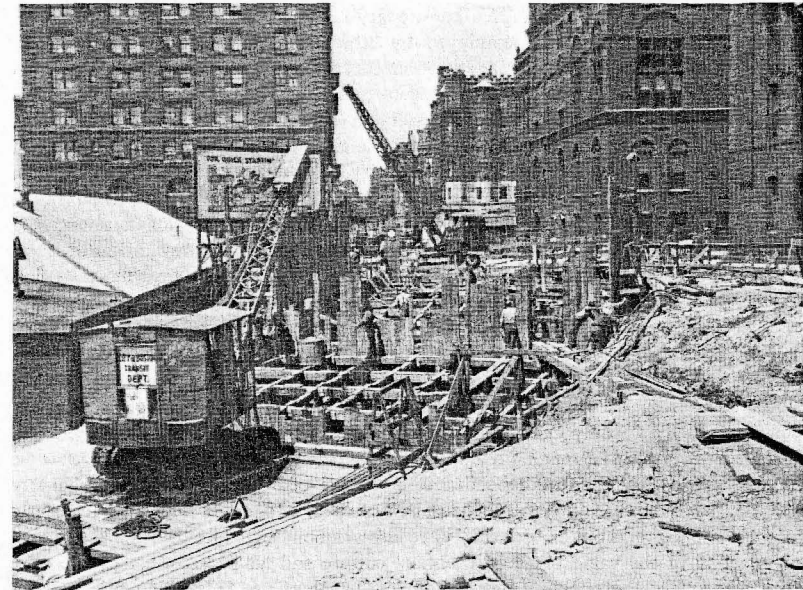
FIG. 3. Construction of the Boston subway system under the Works Progress Administration programme (1938) (courtesy of the US National Archives).
