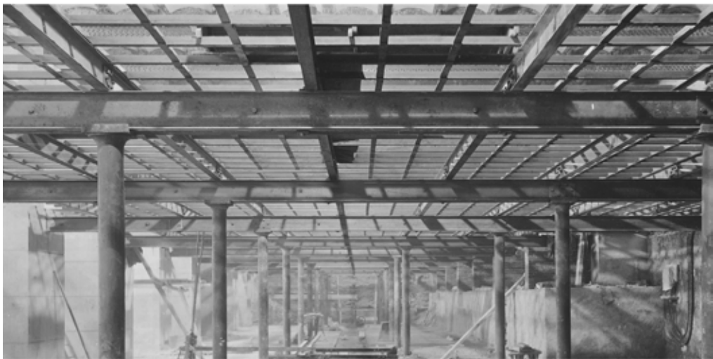
Figure 3. La Samaritaine, Paris. Architect, Frantz Jourdain. Construction of subterranean passageway showing use of steel beams, c. 1905-10. Unknown photographer, La Samaritaine Archives.
